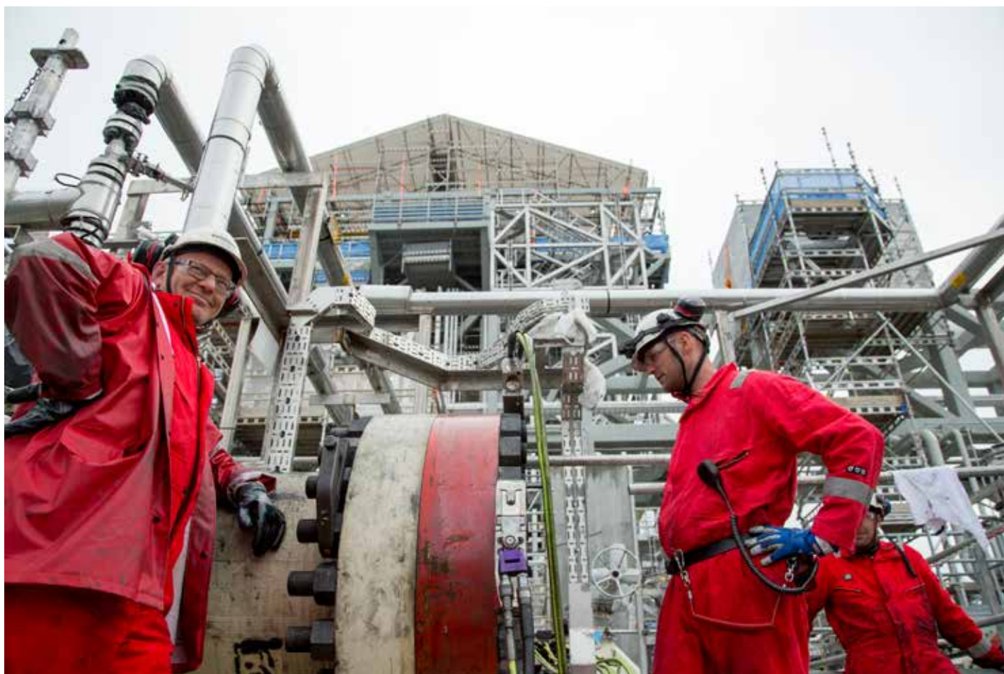
Hooking up. Industrial pipefitters from Kværner put the finishing touches to piping at the receiving module for Aasta Hansteen at the Nyhamna plant. From left: Svein Nygård, Øystein Erland and Stig André Bukkøy.
