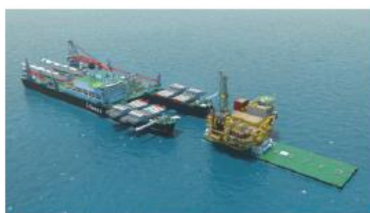
8. The topsides are transferred to the cargo barge and loaded in at the quayside
