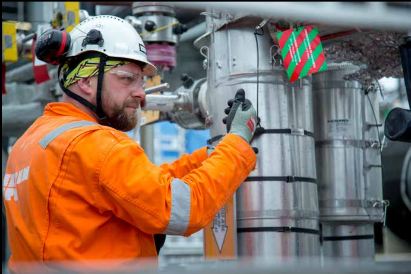
Insulation technician. Krzysztof Mierzwinsky working for Beerenberg on insulating the new reception module for Polarled and Aasta Hansteen at the Nyhamna plant.
